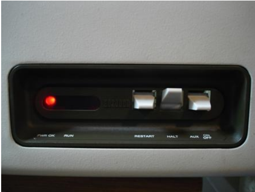
DC Power is OK. System is ready to go!
