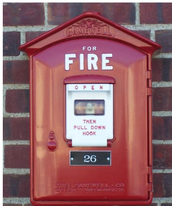
A Gamewell Fire Box Alarm. These use a telegraphic method of signaling that dates back to the 1850's. Obsolete? Perhaps, but you can still buy brand new equipment that works exactly the way it did in the late 19th Century!
