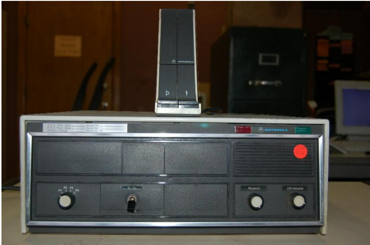
A four-channel Motorola "Super Console" Base Station used for Fire Department and Emergency Medical Service Communications. These base stations date to the mid-1970's.
